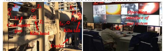
Fig. 11. Installation locations of sensors (left) and the central control room (right).
